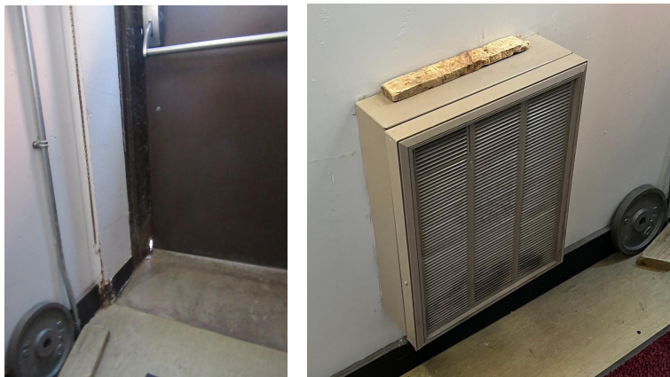
Figure 2: The Degraded Exit Door and the Vent next to the Door
