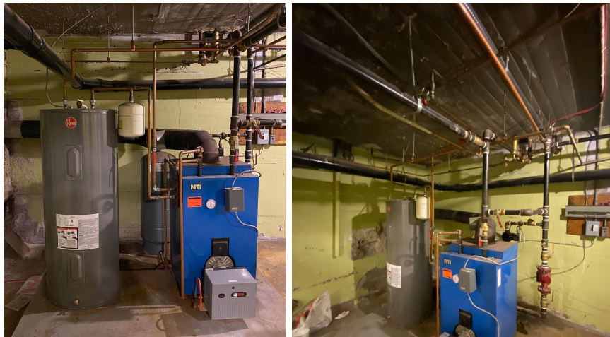
Figure 6: Uninsulated Hot Water Pipes
